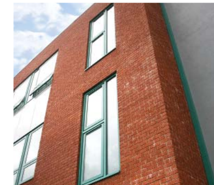
Superlintels with Duragalv 140 (& Duplex finish) were specified as an alternative to stainless steel to meet 60 years PFI design life and exposed soffit application at Northampton School for Girls
